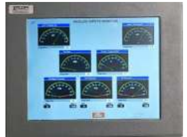
Analog facilities gauges
