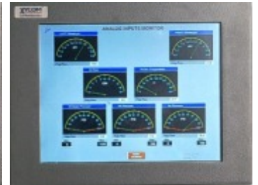
Analog facilities gauges
