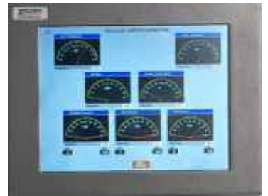
Analog facilities gauges
