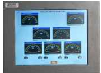
Analog facilities gauges
