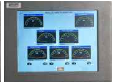
Analog facilities gauges
